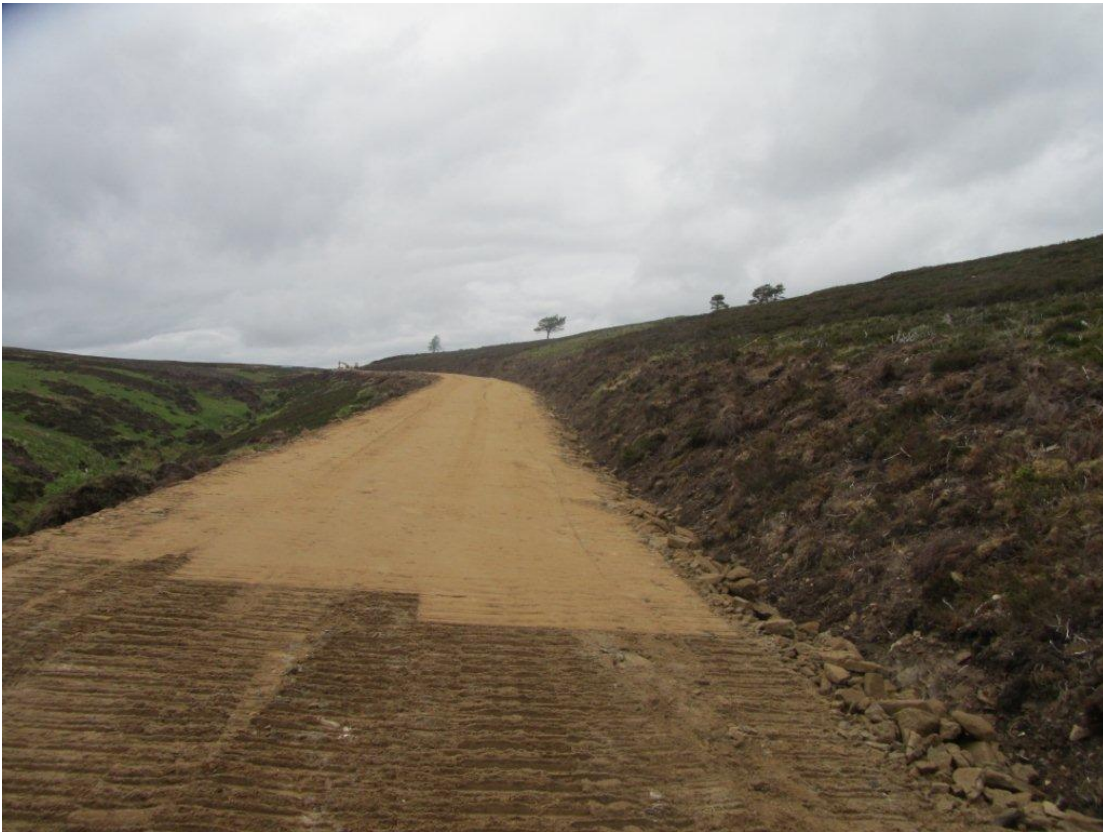
RWE NRL site in Aberdeenshire called Kildrummy. Civils works commenced in May 2012. Picture taken in June 2012 following initial reinstatement of road and verges which utilised peat turves for reinstatement of the verges which were on a 1:1 slope.
