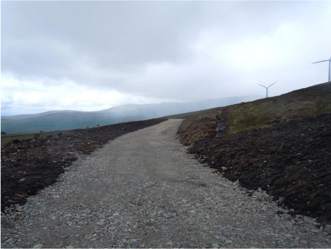
RWE NRL site north of Inverness called Novar 2. Civils works undertaken in summer 2010. Picture taken in late 2010 following initial reinstatement of road and verges which utilised peat turves for reinstatement on the uphill side which was on a 1:2 slope.
